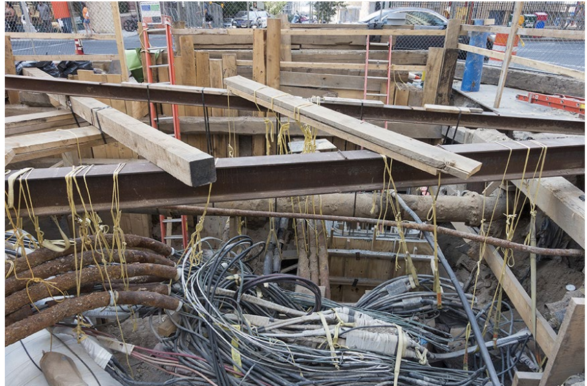
Underground residential lines
