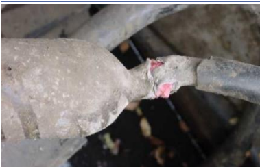
Damaged and leaking cable
