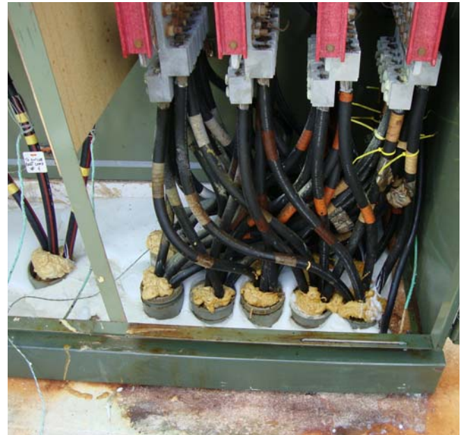
InstaGrout™ Sealant is used to fill a transformer cabinet base in place of concrete.
